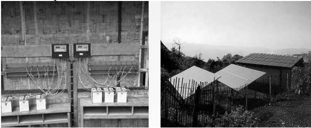
Figure 7: A battery charging station in a Northern Lao village
